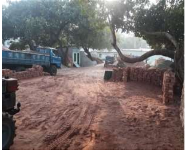
sewage pumping station-2 Motiarkhali khal
