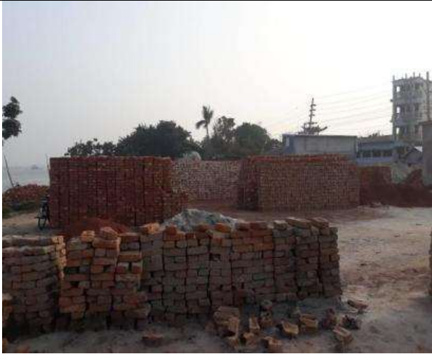
sewage pumping station-1, Customghat
