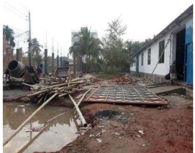
sewage pumping station-6, Truck terminal road, Sonadanga
